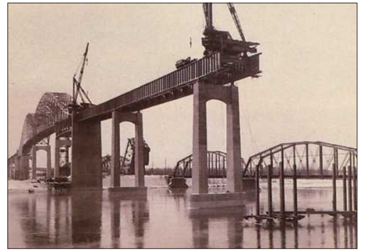
CONSTRUCTION OF the International Bridge took place between 1960-1962. Photo credit: International Bridge Authority
