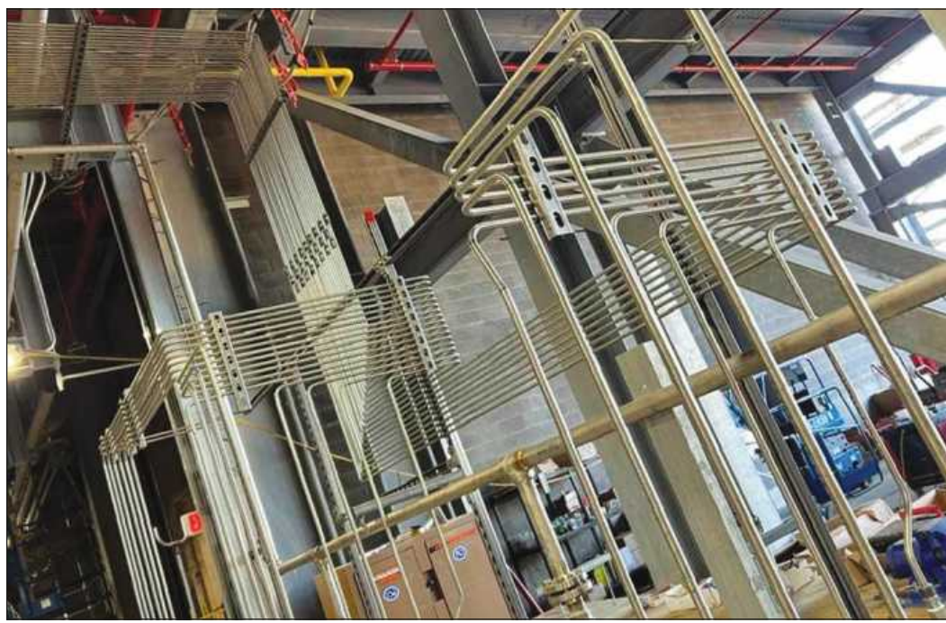
WITH THE COST of the stainless steel pipe "astronomical," according to foreman Johnny Ortiz, the crew had to plot the bends very carefully to avoid waste and pushing up the cost of the project.
