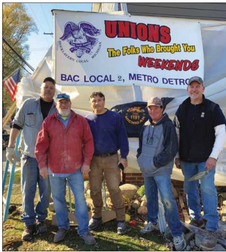
BRICK AND STONE WORK at the Wencel home, as well as interior tile installation, are being contributed by volunteer members of the Bricklayers and Allied Craftworkers Local 2 and Laborers 1191. Shown here (l-r) are Jim Ritchie of BAC Local 2, Scott Redlin (retired Laborers 1191), Raul Zamarrin, Tim Murray, Don Bruning, and (not pictured) Aaron Pistor of Local 2.
